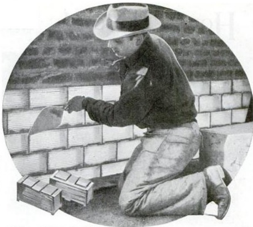
Figure 14 - Installation of glass blocks at the roof of the Barbizon Plaza Hotel (published in "Glass Walls Now Used in Building", Popular Science , June, 1930)
